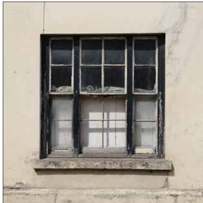
Fig. 7 Original windows should be retained and repaired
