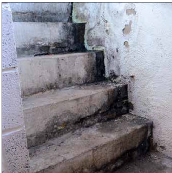
Fig. 9 Water damage to cellar steps in a Listed Building
